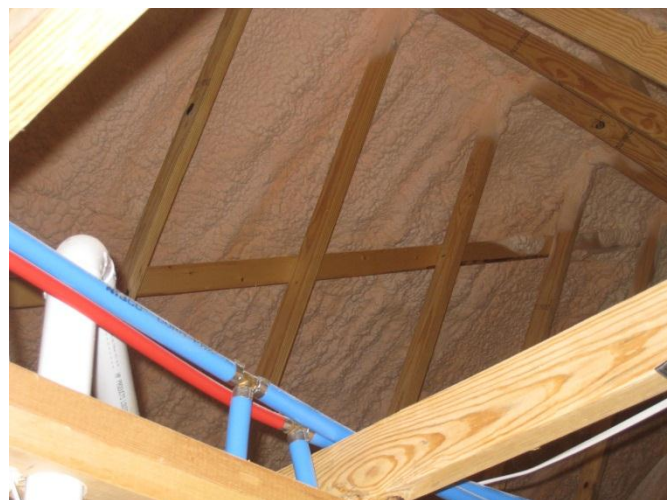
Figure 2 - Spray Foam under a Roof Deck
