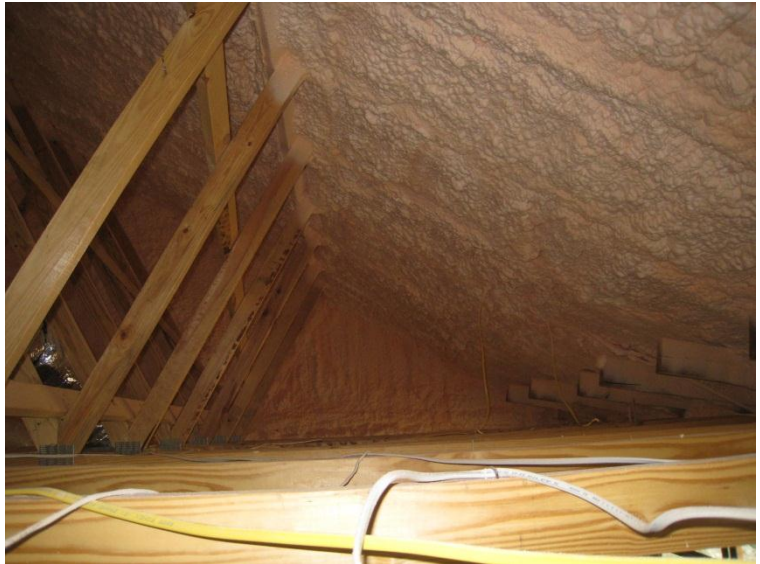
Figure 6 - Spray Foam in an Attic
